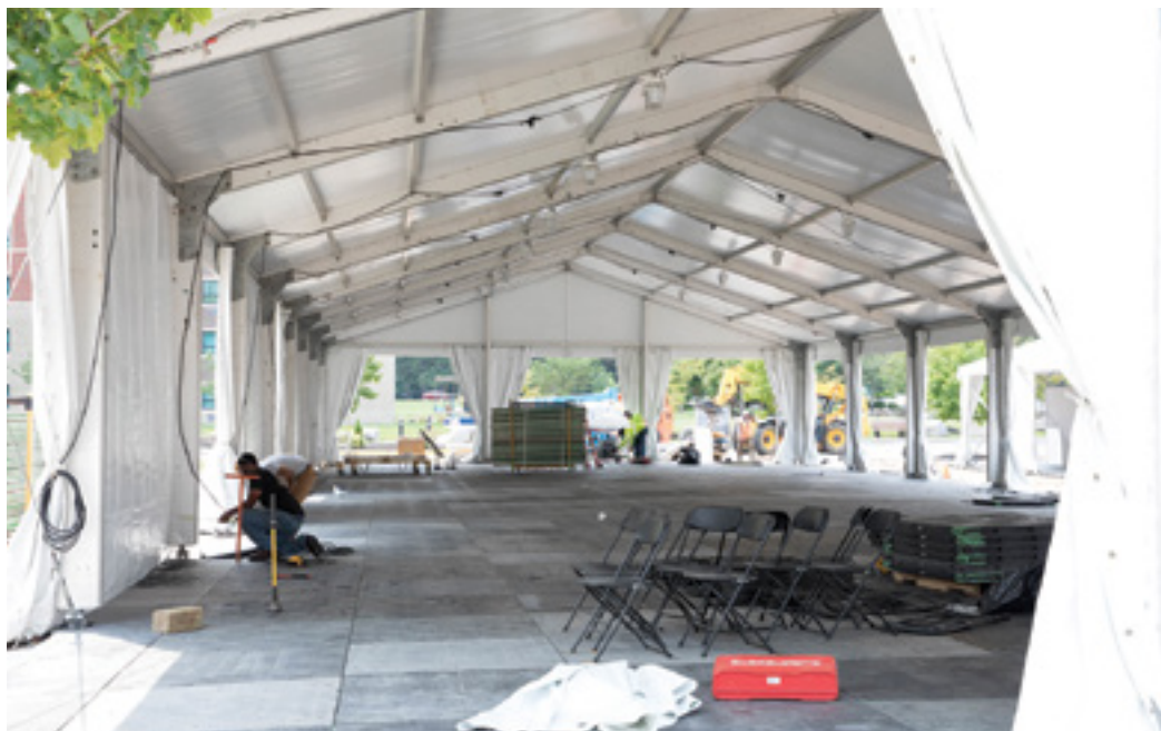
Civilian contractors construct a tent in preparation for the arrival of Afghan special immigrant visa applicants at Fort Lee, Virginia. (U.S. Army photo)
