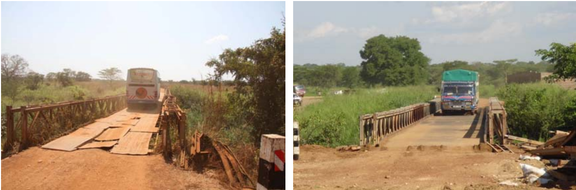
Photographs of Bridge #5 (Kit Bridge) before repair (left) and after repair (right). (The Louis Berger Group, Inc., January 2008.)
