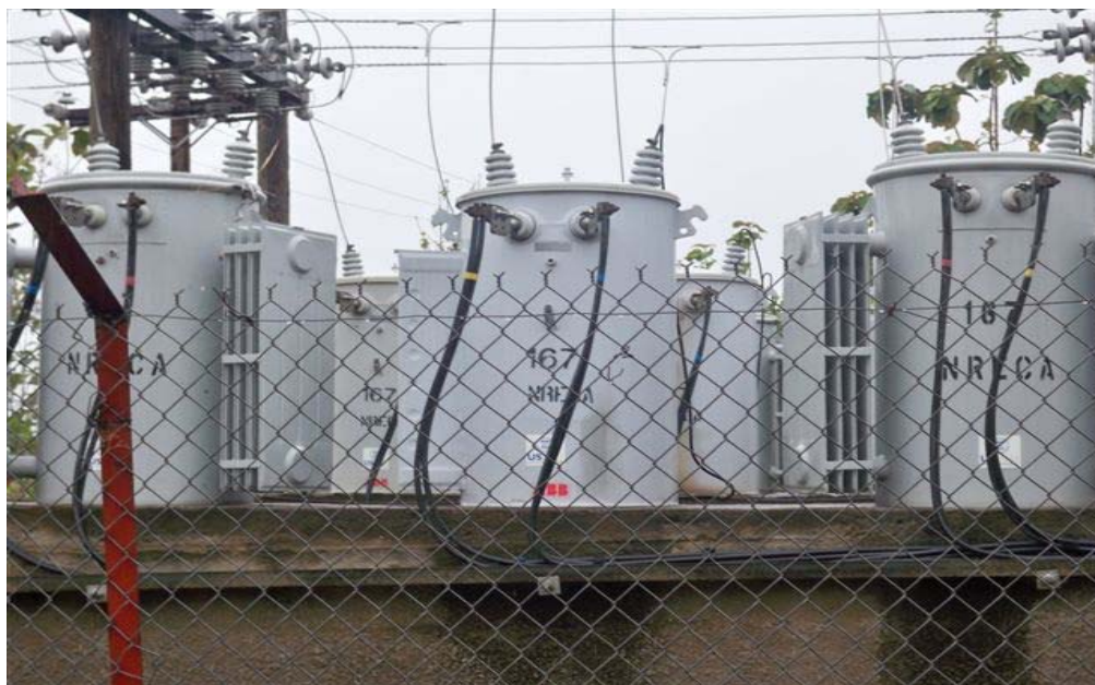
Transformers changing the voltage and/or phase of electricity produced by generators at the Yei Electricity Cooperative in Southern Sudan. (Photo by RIG/Pretoria, February 2010)
