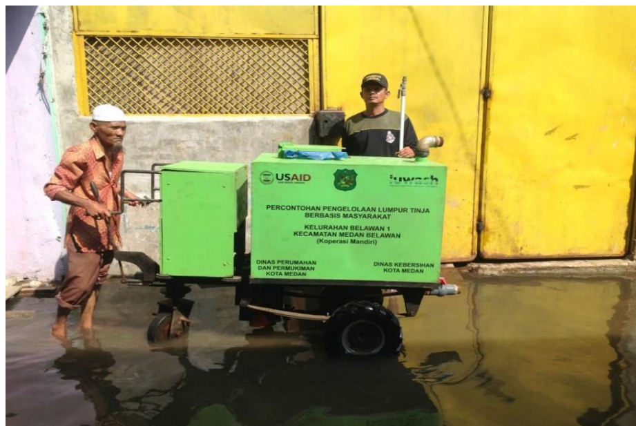
Wading in flooding from a heavy rain, operators in Belawan, Medan, in North Sumatra demonstrate their sludge pumps. (Photo by RIG/Manila, June 13, 2014)
