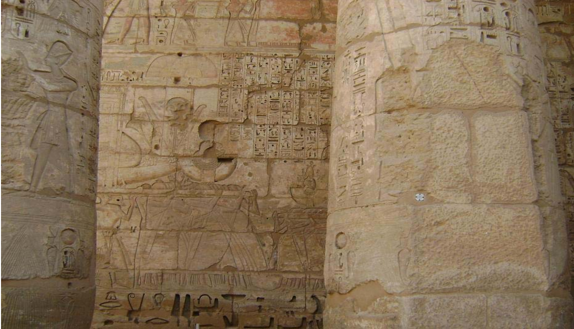
A monitoring point is visible on the column at right in Medinet Habu Temple, Luxor, Egypt. (Photo by OIG, March 2010)
