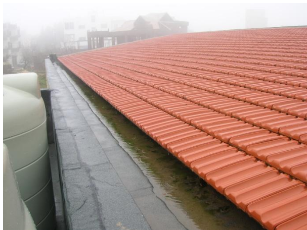
The program rehabilitated this roof at Ehmej Intermediate School in Mount Lebanon. (Photo by RIG/Cairo, February 19, 2013)
