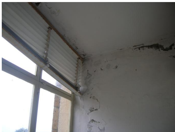
Leaking old windows on the second floor caused water damage to walls and ceilings in the rooms there. (Photo by RIG/Cairo, February 19, 2013)
