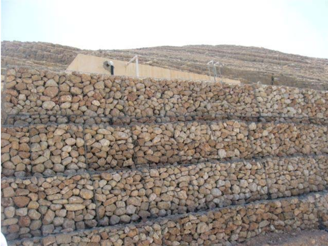
This gabion wall constructed under the Emergency Jobs Program prevents flooding and landslides in Ein Shibly in the Nablus Governorate. This labor-intensive method of construction creates jobs. (Photo by the Office of Inspector General, June 2010)
