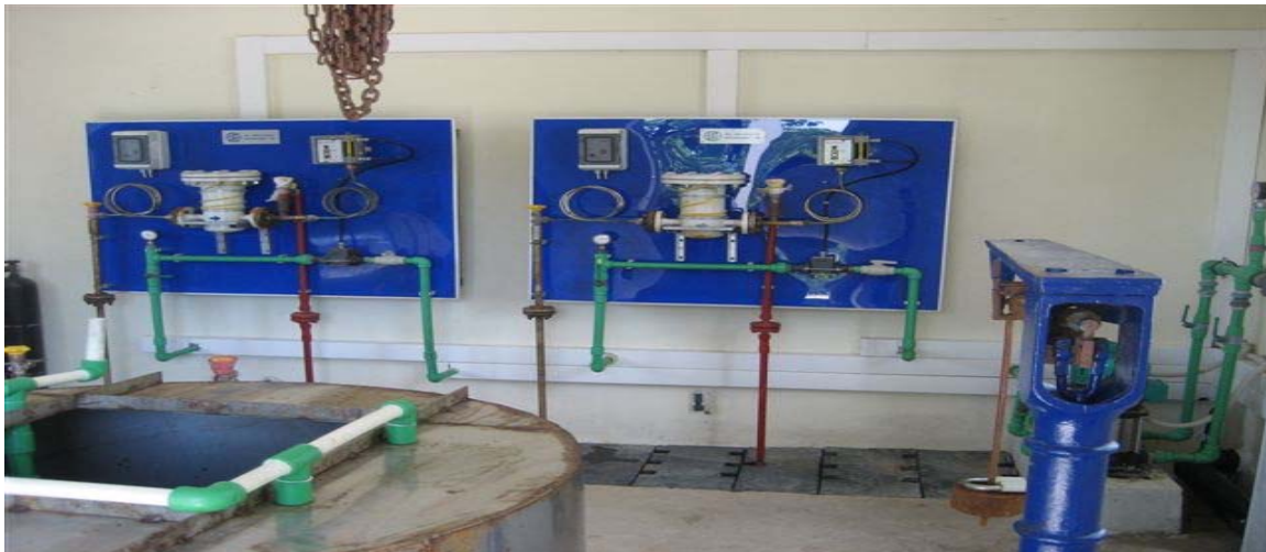
Photograph of new chlorination plant in Poti, Georgia, taken by OIG Auditor on June 1, 2009.
