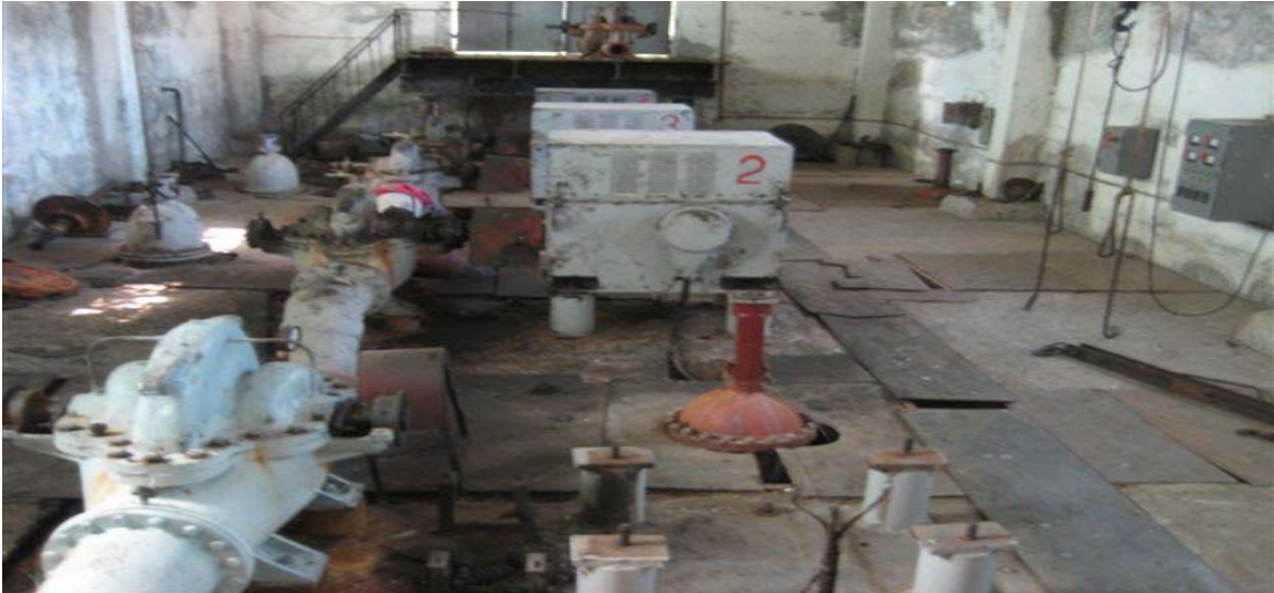
Photograph of Old Soviet Pumping Station in Kutaisi, Georgia, taken by OIG Auditor on June 2, 2009.
