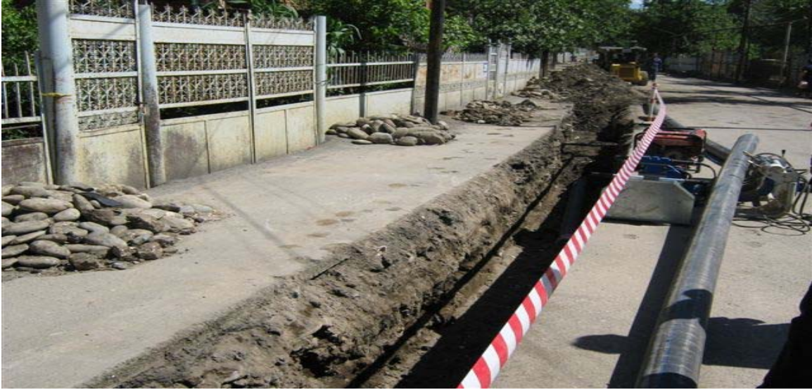
Photograph of new pipe being laid in Kutaisi, Georgia, taken by OIG Auditor on June 2, 2009.
