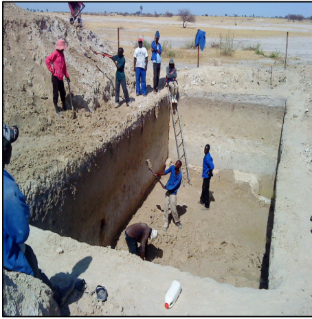
This photo documents conditions reported by supervisory engineer prior to the OIG visit. OIG also observed workers without protective equipment and open trenches without barriers. (Photo by supervisory engineer, December 2010)
