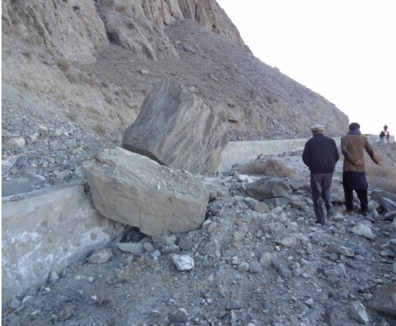
These boulders are crushing the wall of one of the two main canals. Photo: OIG (December 21, 2015)
