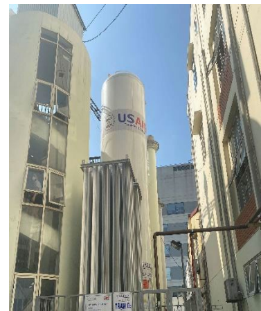
USAID-funded liquid oxygen system located at Long Khanh Regional General Hospital in Dong Nai, Vietnam (photo by Williams Adley)
