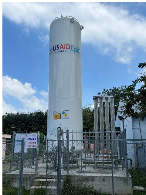
USAID-funded liquid oxygen system, under a separate CN, located at Long Khanh Regional General Hospital in Dong Nai, Vietnam (photo by Williams Adley).
