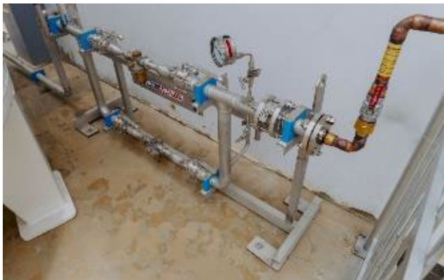
Liquid oxygen piping for LOX system in Vietnam, funded under a separate CN (photo by Williams Adley).
