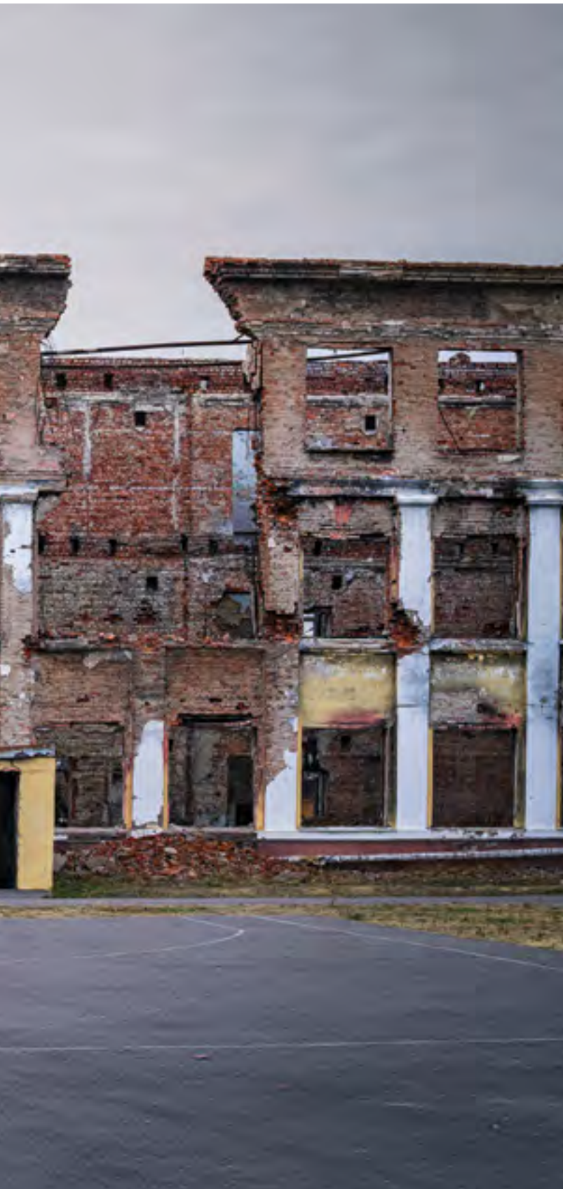
A destroyed school building in Kharkiv. (WFP photo)
