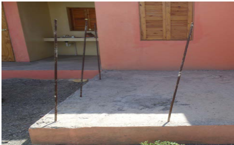
Reinforcing bars on open slab intended for future expansion pose a safety hazard in Caracol-EKAM. (Photo by RIG/San Salvador, July 1, 2013)
