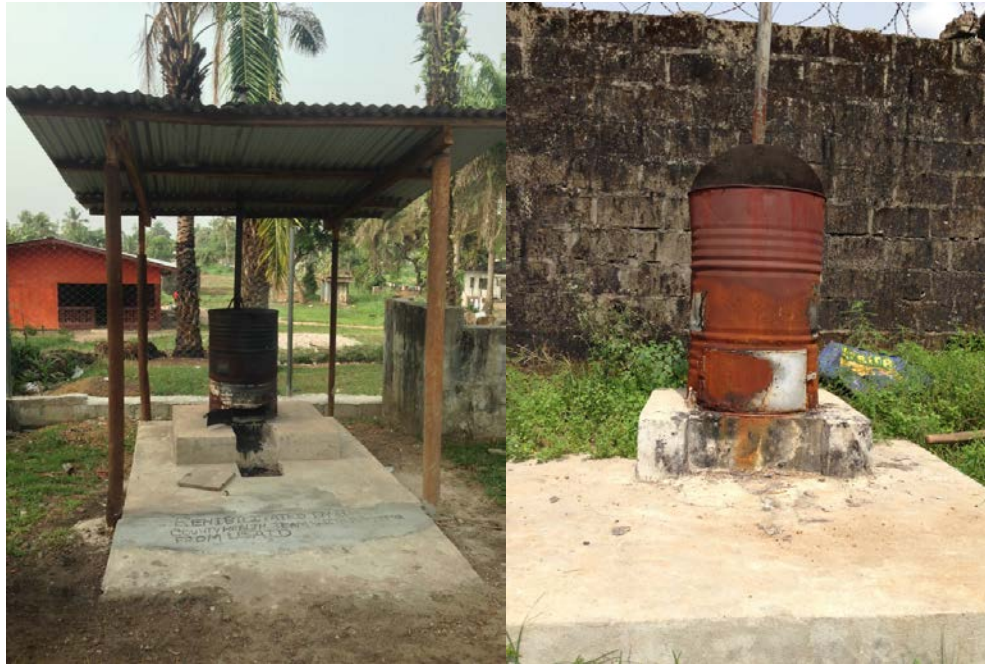
The incinerator at left (Incinerator 3) is oxidized and was expected to cease operating by September 2016. The incinerator at right (Incinerator 4) is no longer operational, and the facility was burning waste beside it, close to the clinic entrance. Photos: OIG (January 27 and 28, 2016)
